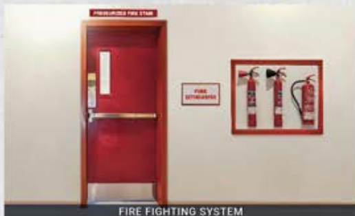
FIRE FIGHTING SYSTEM
